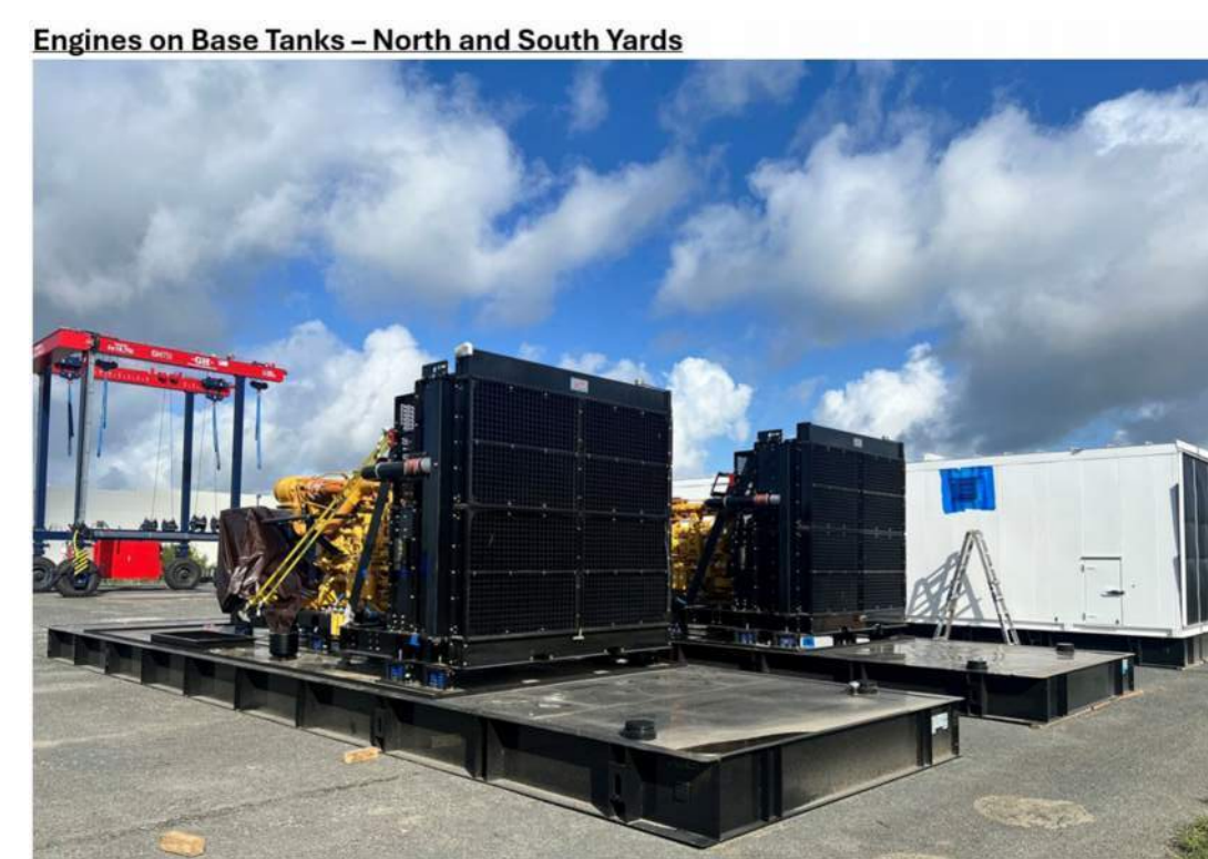
Engines on Base Tanks - North and South Yards
